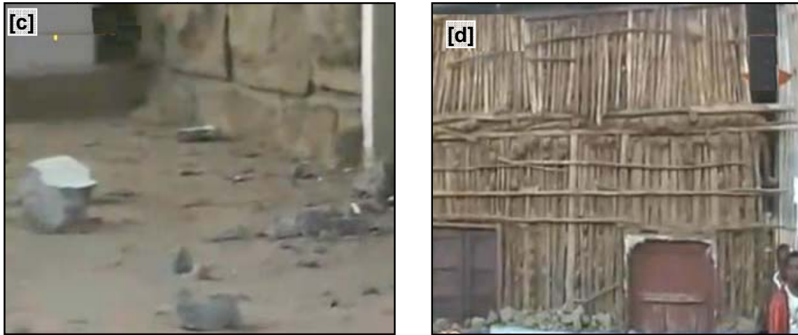
Figure 6 Photographs of structural damages due to the December 2010 Hossana earthquake. [a]-[c] show damages to reinforced concrete frame dormitory buildings at Jimma university where 26 students were injured. [b] structural damage to slab and column joint. [c] debris from damaged frame. [d] damage to the masonry clad of a timber building. EBCS-8:1995 classifies Jimma as seismic zone 1. (Image Source: Ethiopian TV.)
