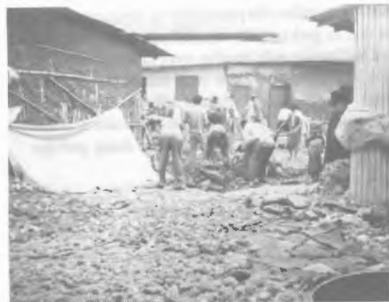
Plate 4: Compound paving (Note the "bikil" production and the half barrel in the foreground)
