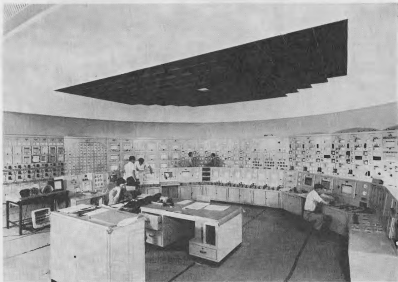
Fig. 3 — The control room of the C.E.G.B. Nuclear Power Station at Bradwell
