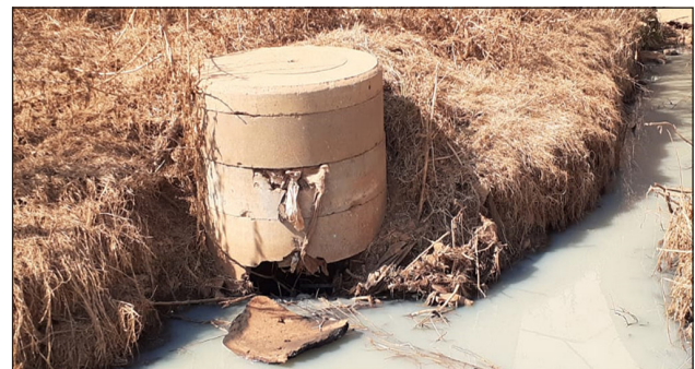
Figure 1. Vandalized sewer manhole in the study area
