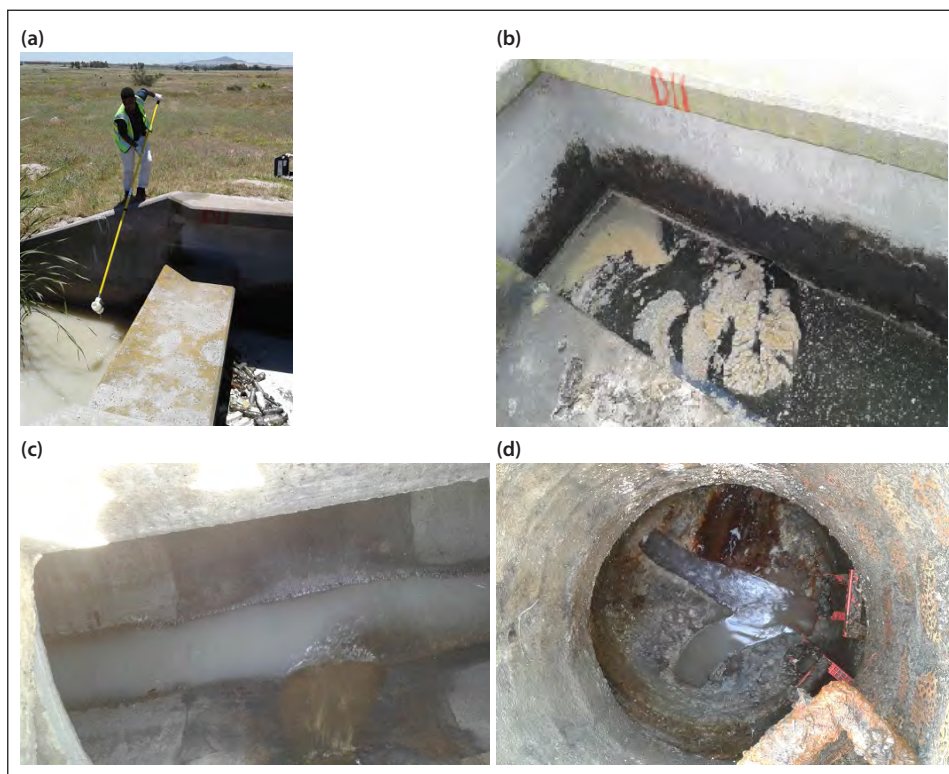
Figure 10. Photos of illegal discharges traced from Outfall D11 to source: (a) white milky colour flow – Outfall D11; (b) white spoiled milk floatables – Outfall D11; (c) white milky flow – manhole; (d) white milky flow – manhole
