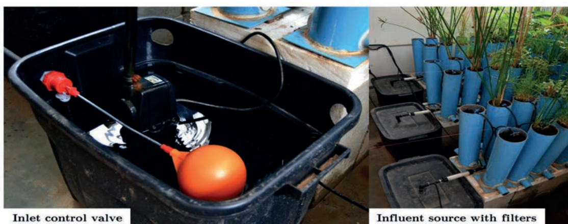
Figure 3. Flow inlet control and submersible pump and a depiction of the irrigation filters
