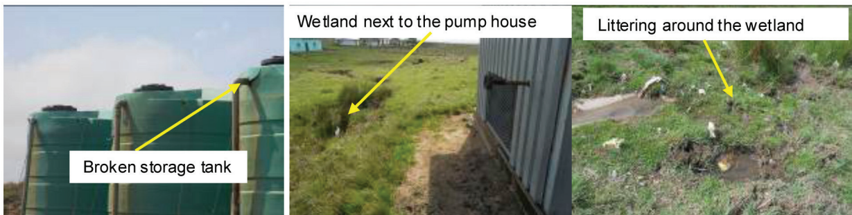
Figure 4 Case Study 1 on-site observation issues noted
