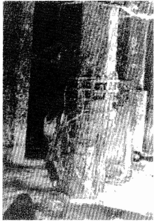
Plate 3. Exposed reinforcement in one of the piers at main quay
