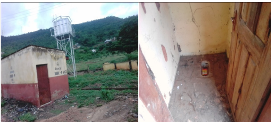
Figure 2: Non-functional 4-pour flush toilet facility in Kabawa community
