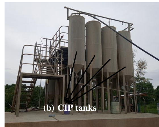
Figure 14: (a) Ball mill (b) CIP tanks at Itumbi mineral demonstration centre.
