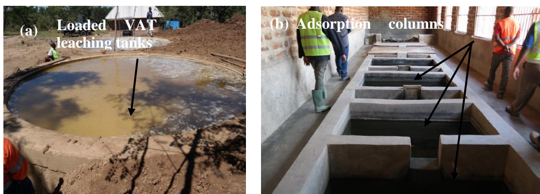
Figure 12: (a) VAT leaching tanks and (b) Carbon adsorption columns.
