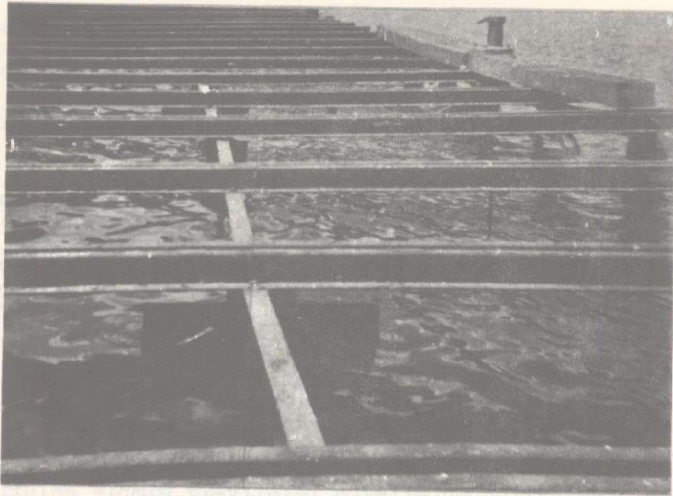
View on Jetty Steel Substructure after removal of timber deck. 20th June, 1972.
