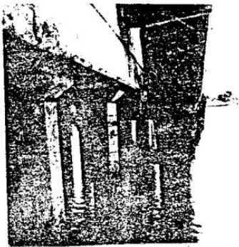
Fig. 8 Broken off fender system due to corrossion of support areas
