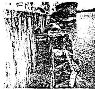
Fig. 7 Corrosion of steel bars in concrete piles at the port area
