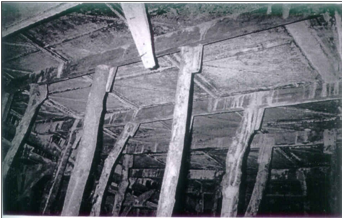
Fig. 1: One of the typical construction sites with “Mirunda” formwork supporting a reinforced concrete slab.
