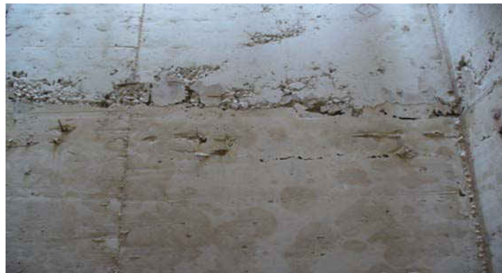
Figure 3. State of reinforced concrete shear wall at one of the sites.
