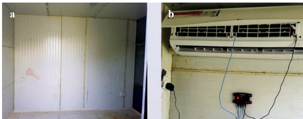
Figure 1: Wall insulation in a cold room (a) and a CoolBot mounted on an air conditioner in a cold room (b) at the Horticulture unit in SUA, Morogoro, Tanzania.
