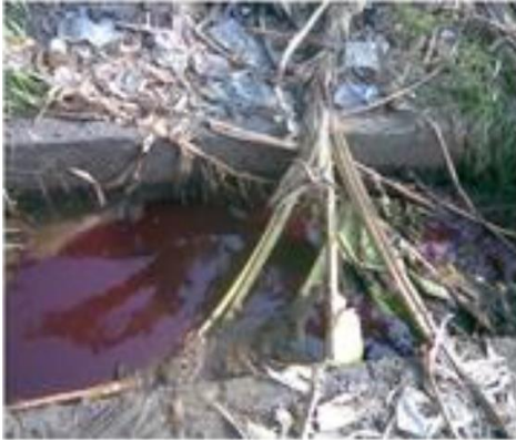
Plate III: Blocked drainages within the slaughterhouse facility
