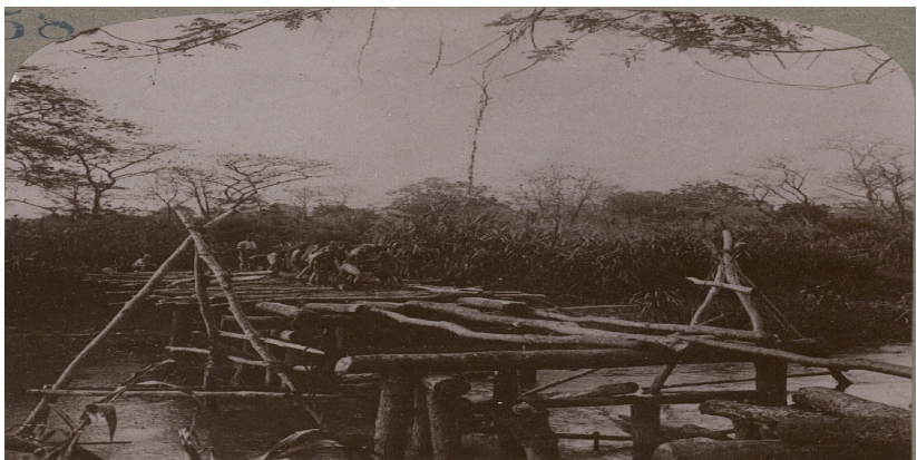
Figure 2: Bridge construction over the Mgeta River in German East Africa, 27 August, 1916, by permission of the Centenary of World War I in Orange, Orange City Council. A rudimentary bridge under construction.
