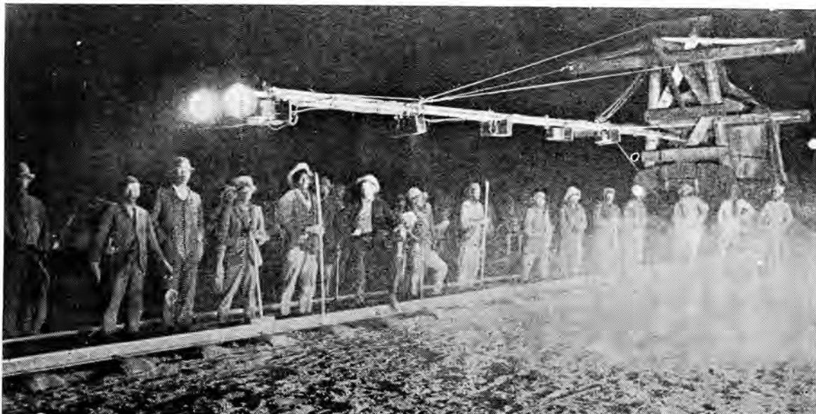
The mobile plant which enabled work on the Prieska-Upington line to proceed at night
