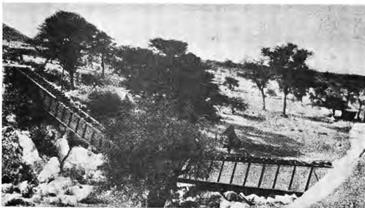
A frequent sight: demolished bridge, GSWA
