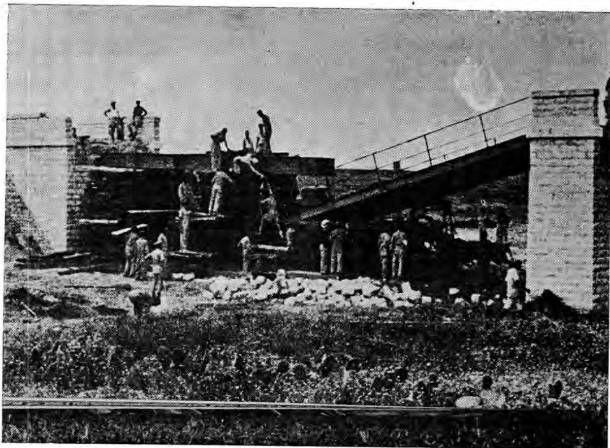
A damaged bridge on the Western Desert Railway
