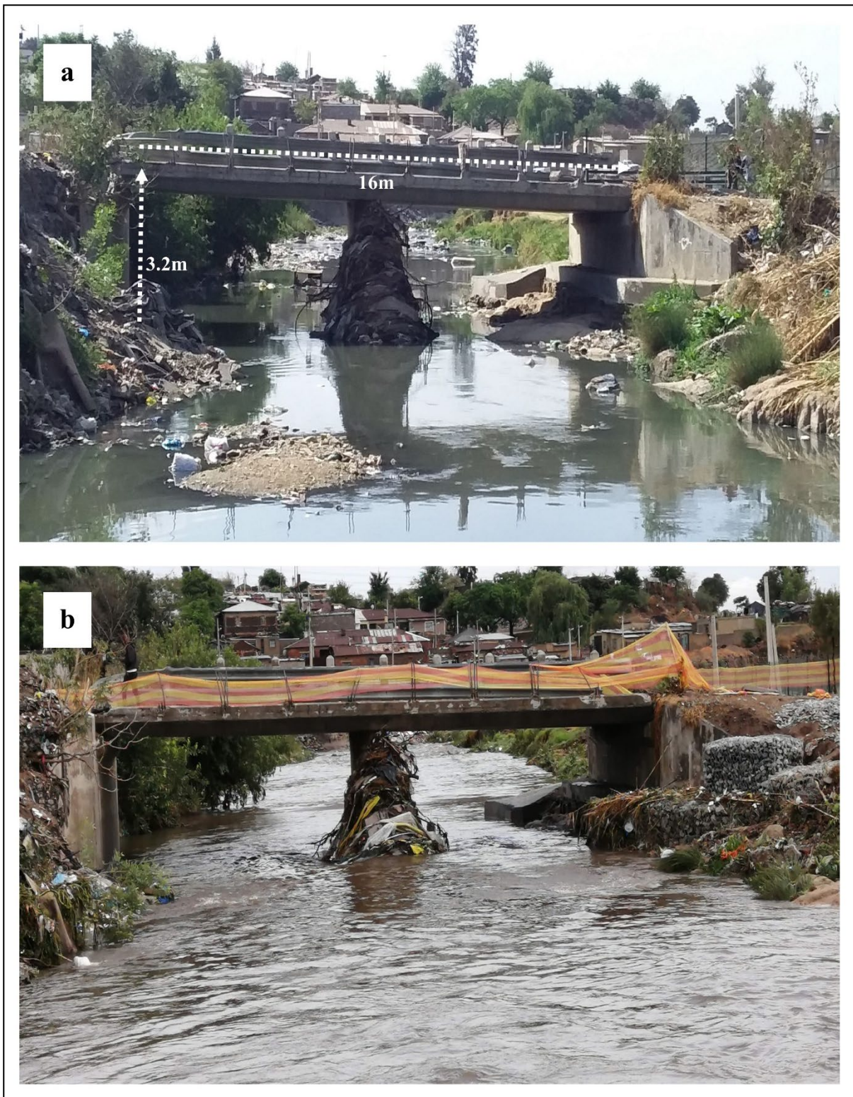
Figure 12: Photographs of a bridge (a) during the normal period and (b) during the rainy season
