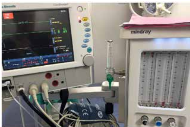
Figure 1: Anaesthesia workstation being tested after the event; connected to faulty wall gas outlet and ventilating a test lung. While supplying only medical air, note the lack of oxygen or other gas on the analyser display, subtle high flat line EtCO 2 trace and lack of capnograph reading.
