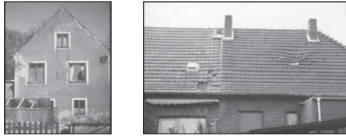
FIGURE 2. Typical example of building class #3 consisting of ‘unreinforced masonry, with load bearing wall, low rise’. Source: EMS98 (op. cit.)
