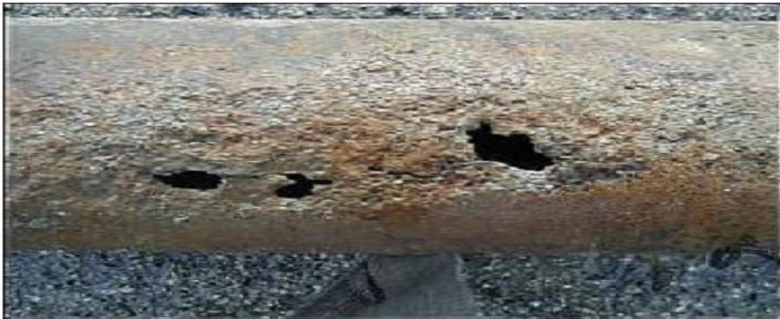
Fig. 2: Corrosion in oil/gas pipeline
