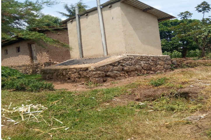
Figure 4. 1. The Ecosan technology/UDDT constructed by SNV at household in Rugarama Sector.
