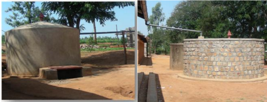
Figure 3.Up ground tank - Model 1 and 2 (Murama Primary School)
