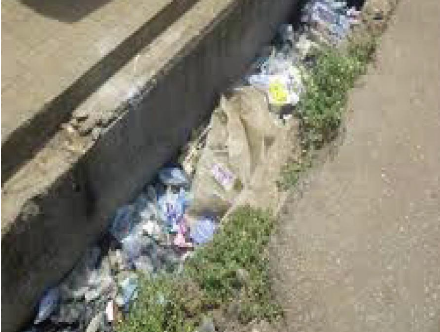
Figure 3: Blocked drain a Ghanaian city
