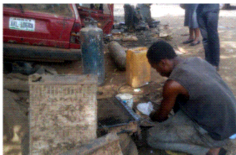
Picture 2: Welder working without protective goggle
