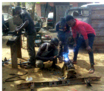
Picture 1: Apprentice learning without protective equipment
