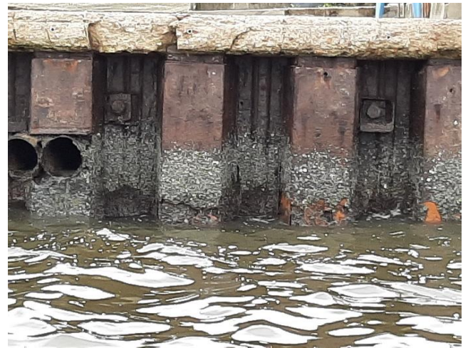
Figure 2: Corroded Sheet pile on the lagoon.
