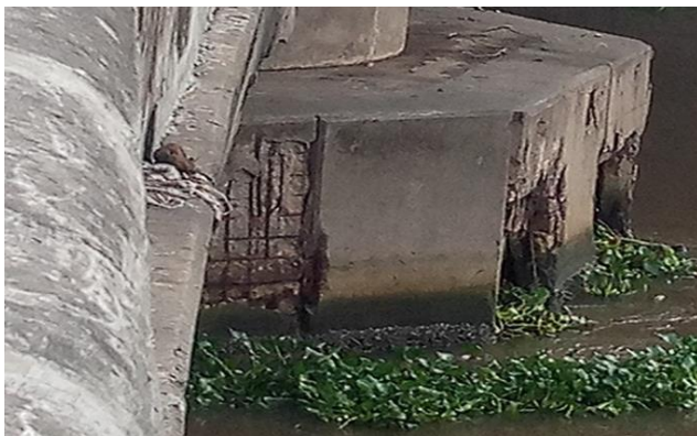
Figure 1: Corroded Reinforcement in Concrete.
