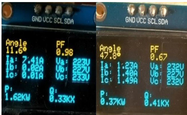
Figure 19: LCD display showing the display output parameters when the SVC is switched ON at no load
