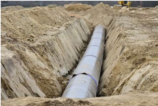
Figure 3: Pipelines buried underground. Source: Author's research.
