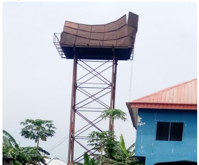
Figure 2: Elevated steel water stanchion.
