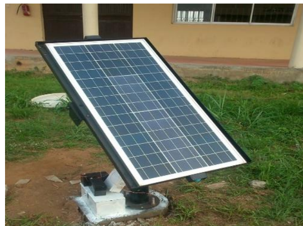
Fig. 14: Solar tracking rack system
