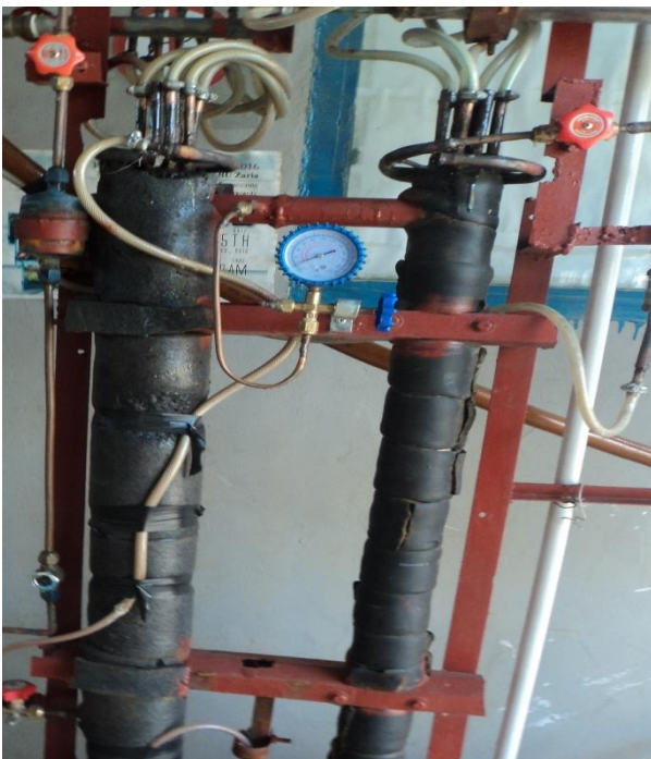
Figure 4: Close up view of Absorber and Evaporator
