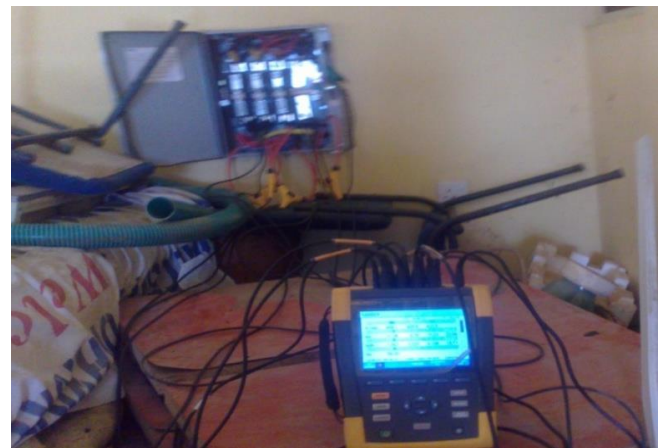
Figure 4: The setup of the Electrical Load Consumption Measurement using FLUKE 434 Series II Energy Analyzer
