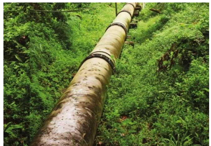
Figure 1: Pipeline external corrosion [4]
