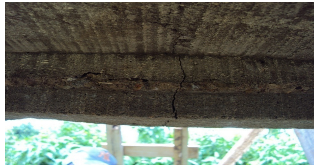
Plate 2: Crack at mid-span of space-framed beam (model B)
