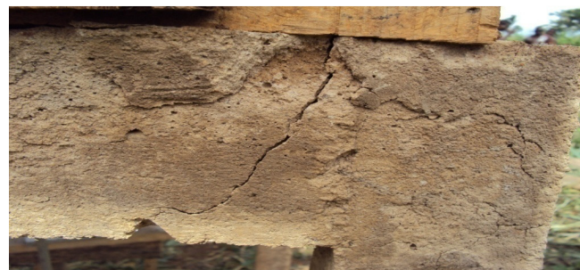
Plate3: Crack at the beam-column joint of space-framed (model B)
