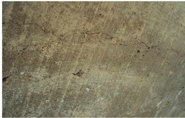
Plate1: Crack at the bottom of space-framed slab (model B)
