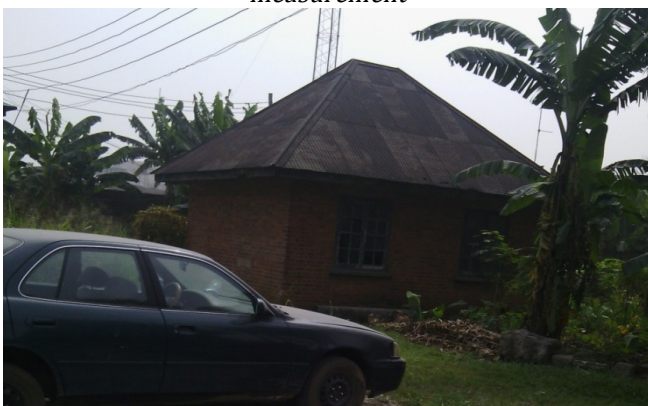
Figure 3: Mud House with Rusted Corrugated Iron Roof Sheet
