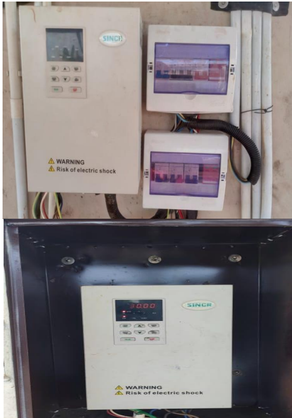
Figure 11: Solar pump inverter during operation.
