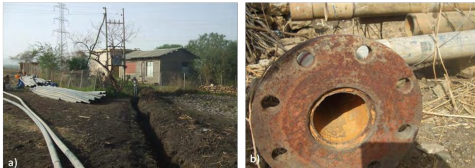
Figure 11. a) Metallic pipes being replaced by PVC after leakage and clogging problems, b) corrosion problem on metallic pipe joints.
