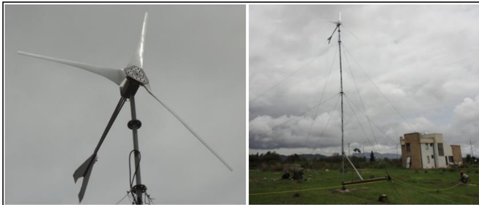
Figure 18. The overall setup of the wind turbine and control room.
