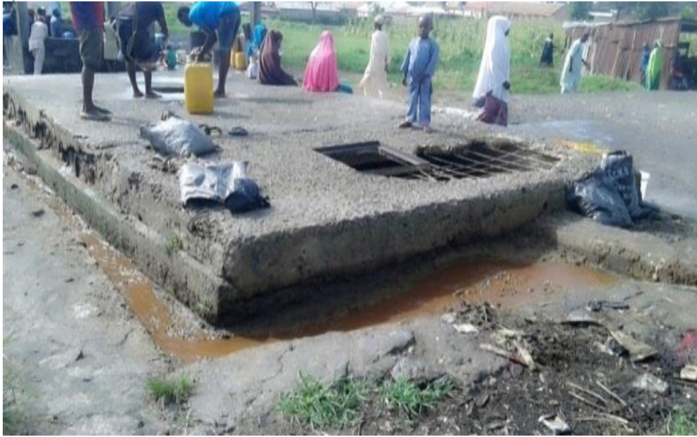
Figure 4. Waste discharged into the environment due to damaged abattoir waste tank. Source: Authors' Fieldwork (2017)
