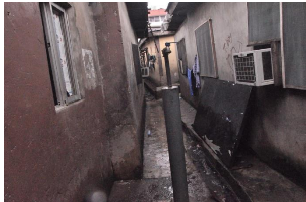
Figure 10: Borehole Water Supply in the Area
