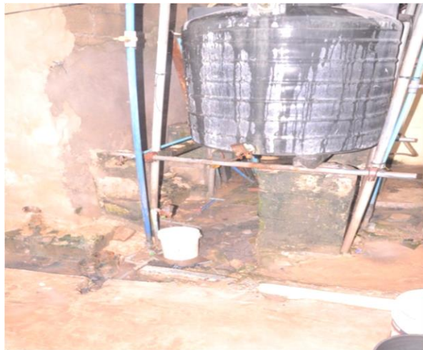
Figure 11: Storage tank for Supply of Water
