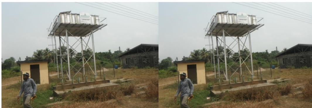
Figure 2: Moribund borehole project depicting poor water supply in the study area Source: Authors' Field Survey, 2020
