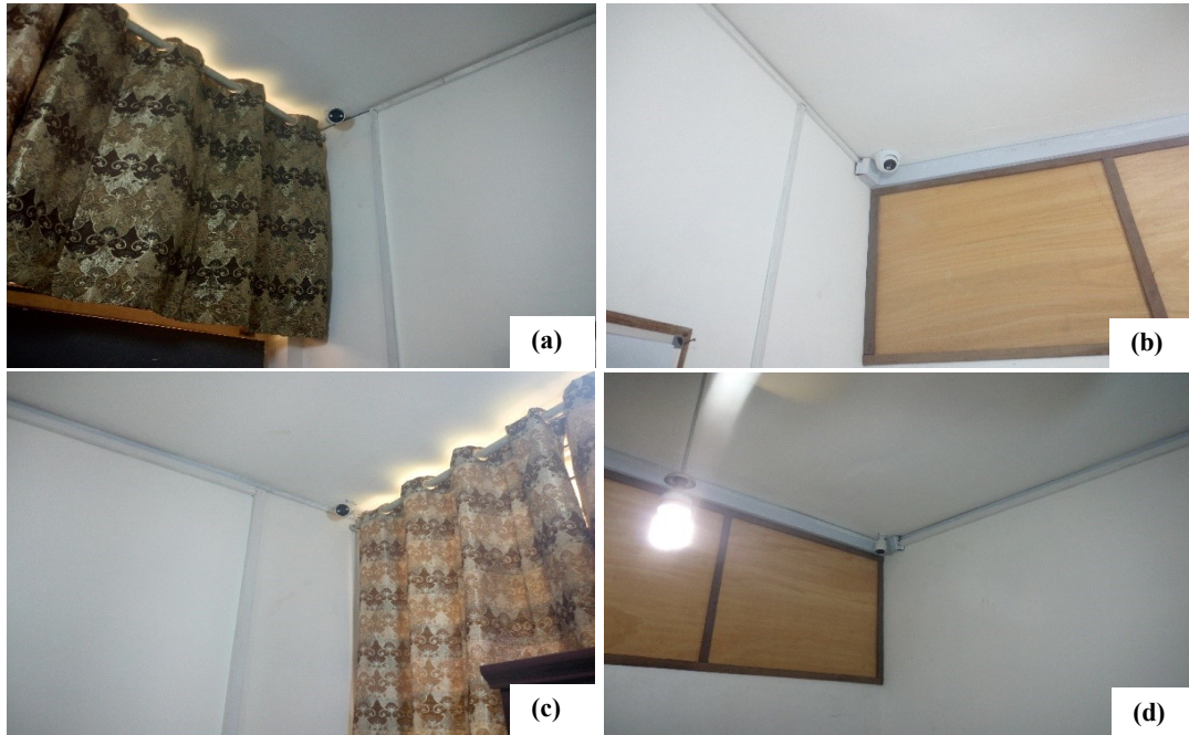
Fig. 2: Four installed CCTV cameras (a) Front left corner camera; (b) Front right corner camera; (c) Back left corner camera; and (d) Back right corner camera
