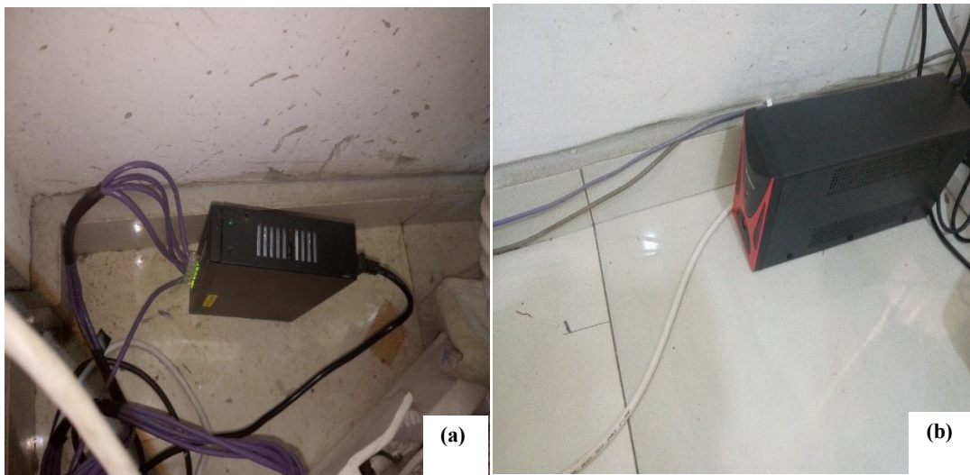
Fig. 4: (a) Installed eight pin switch board for the CCTV; and (b) Uninterrupted Power Supply (UPS)
