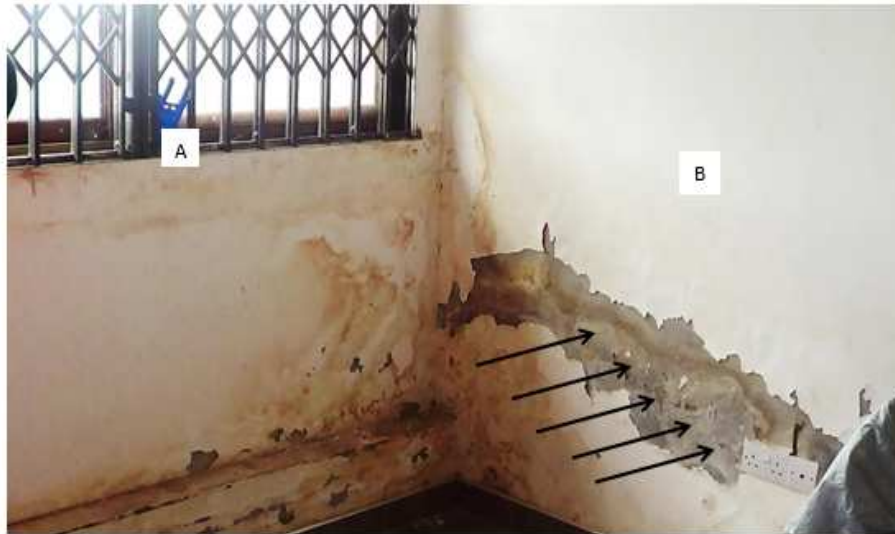
Fig. 8: Stains on internal walls of bedroom 1 (A) and partition of bathroom and bedroom (B)
