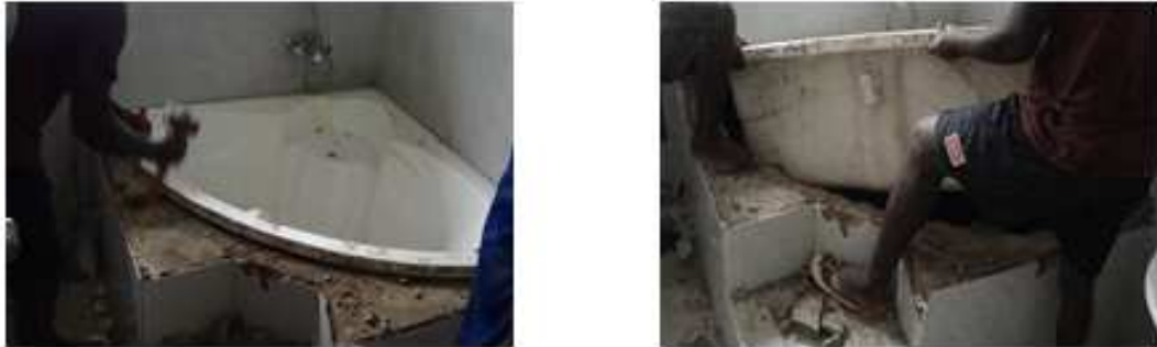
Fig. 22: Tiled walls of the bath tub had to be hammered to pieces to enable the defective bath to be removed
