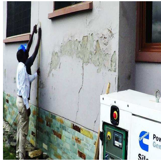
Fig. 7: Western orientation-Dampness measured up to 1.2 m on external walls of bathroom
