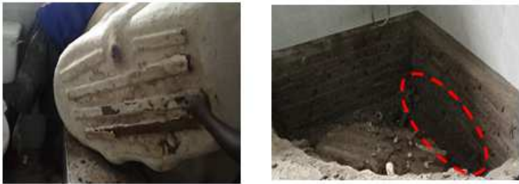
Fig. 23: Conditions at the base of the bath tub after it was removed
