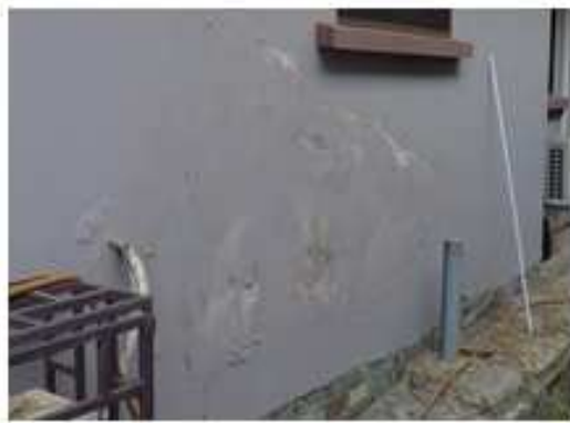
Fig. 21: Dampness on external wall of master bathroom
