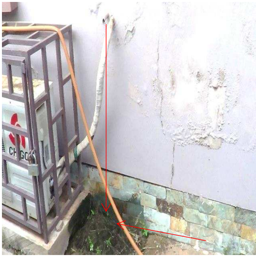
Fig. 6: Water from air condition dripped against the base of wall
