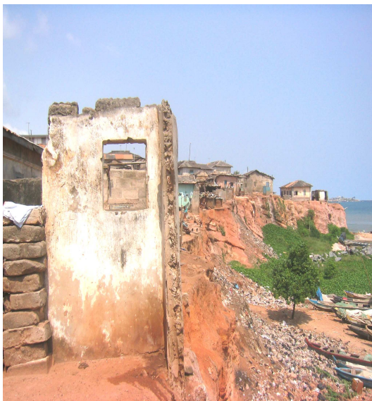
Plate 5: Damaged walls and exposed foundations of buildings
