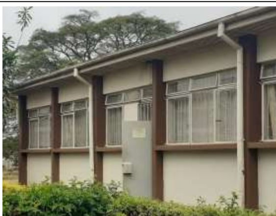
Plate 1: Gutters and discharge pipes, but no tanks on a newer building at main campus
