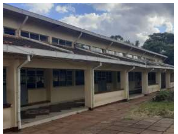
Plate 2: Gutters and discharge pipes, but no tanks on an old building at main campus
