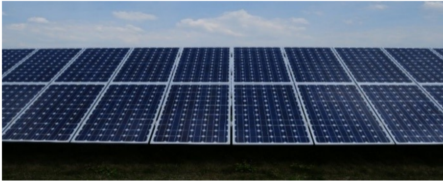
Figure 5 Monocrystalline solar PV array
