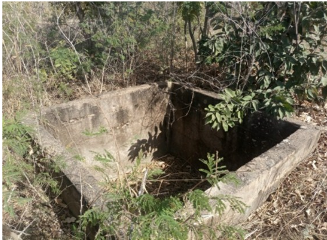
Figure 6 A concrete tank not receiving water due to broken pipe network at the Pulima irrigation scheme
