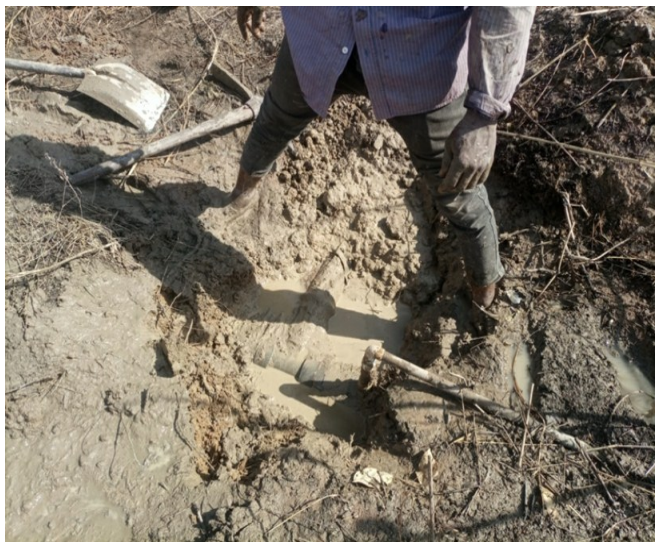
Figure 7 Assessment of broken down pipes to tanks at the Pulima irrigation scheme
