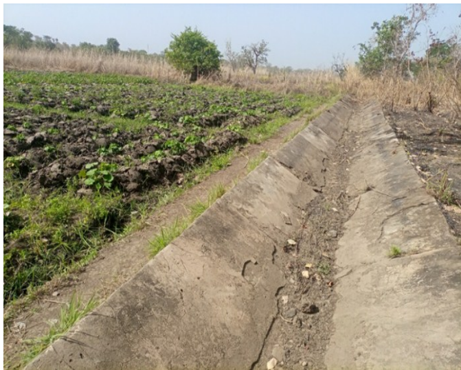
Figure 11 The main conveyance with the canal lining removed at the Yeleyiri irrigation scheme
