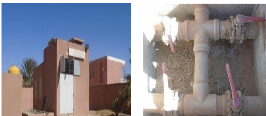
Fig.3. Pumping Station and Repeater
